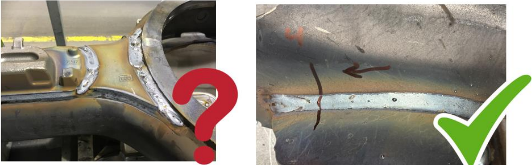
Figure 19. Welds on the rear axle: needing adapted programming (left) and direct scans OK (right).
