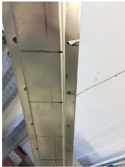
Picture 4: Test specimen that has lost the stiffness caused by cracks round the spot welds.
