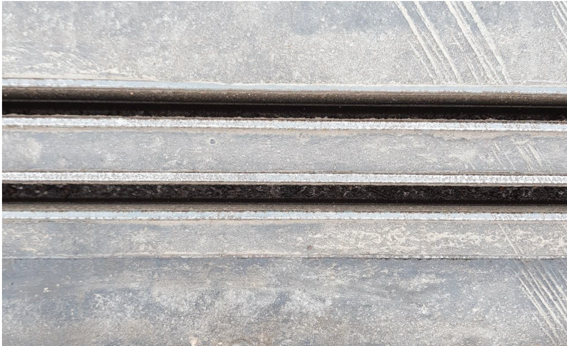
Figure 25: Wear on the ERS conductive rail.
